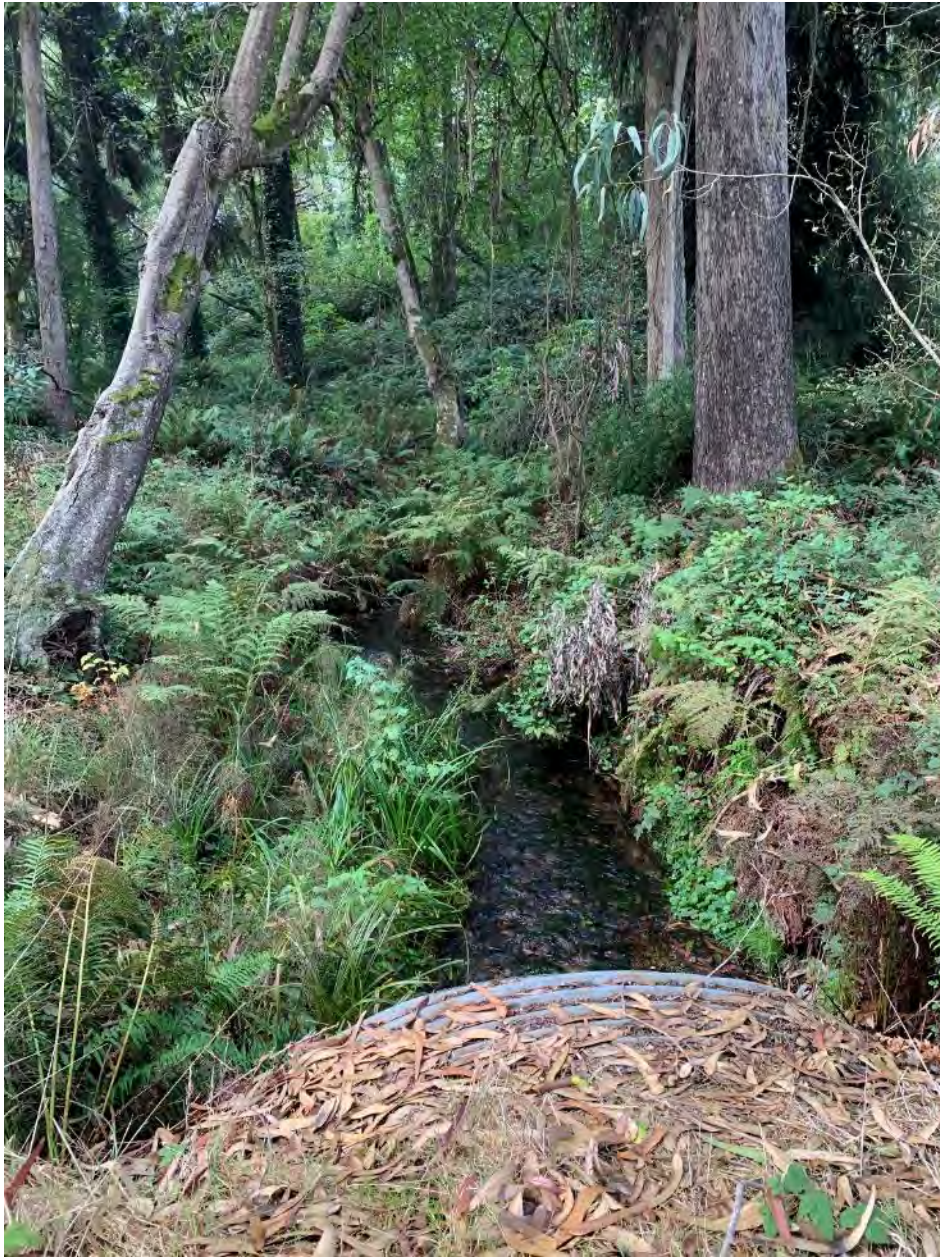
Photo 3. A perennial stream passes through a large culvert under the access road at the confluence of Norton Creek and Widow White Creek. (Highway Crossing Project)
