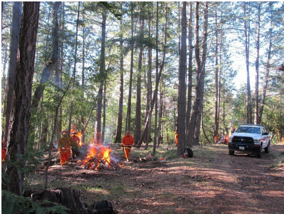
Figure 11 Example of a shaded fuel break on the Soquel Demonstration Forest Santa Cruz County.
